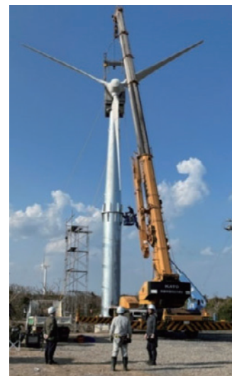
Fig. 16 Wind turbine generator
