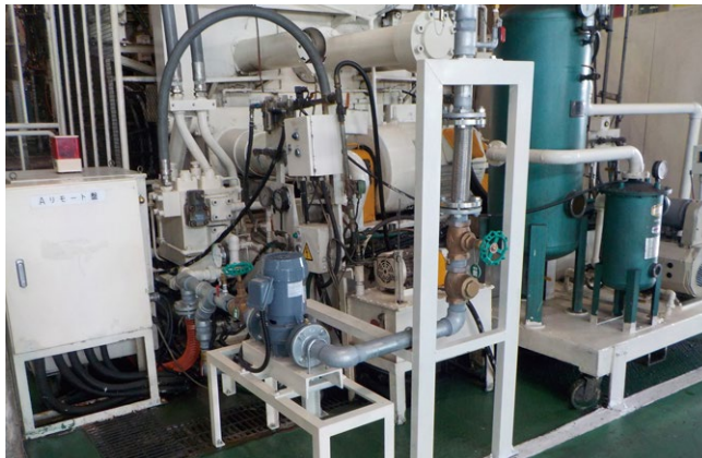
Cold water circulation equipment at forging facilities
